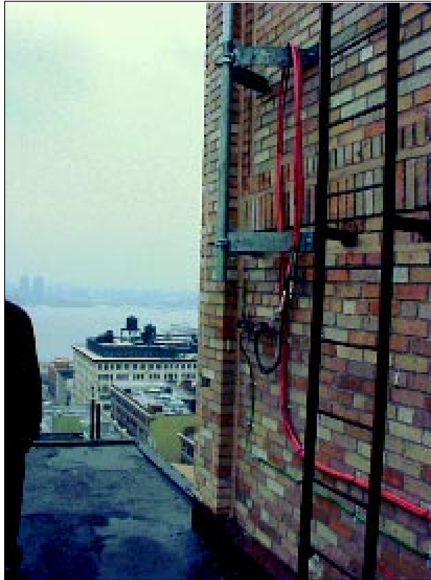
Antenna sites are at a premium in urbanized areas such as New York City. This 14-story rooftop installation is cabled to a base station in the basement.
